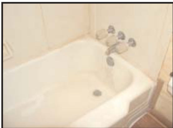
UGLY, UNSIGHTLY, PEELING PAINT
