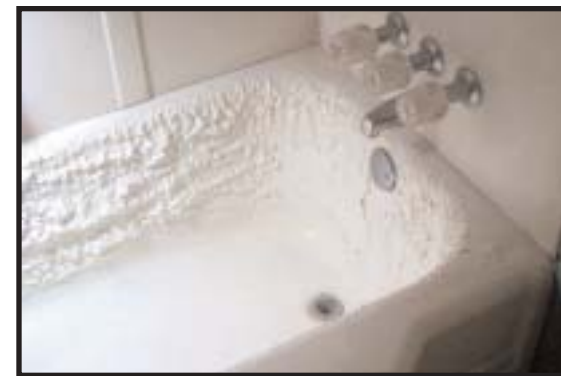
PAINT BEING STRIPPED OFF TUB
