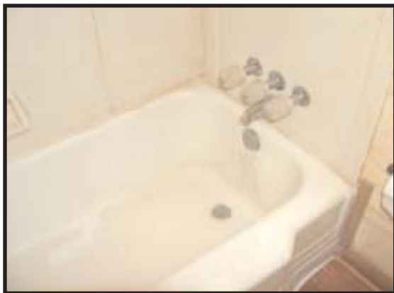
UGLY, UNSIGHTLY, PEELING PAINT
