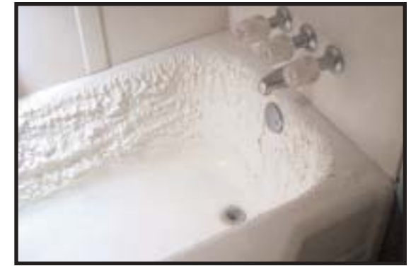
PAINT BEING STRIPPED OFF TUB
