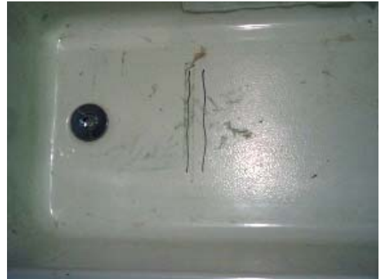
Close up of a cracked area
