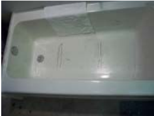
Cracked tub bottom in two locations
